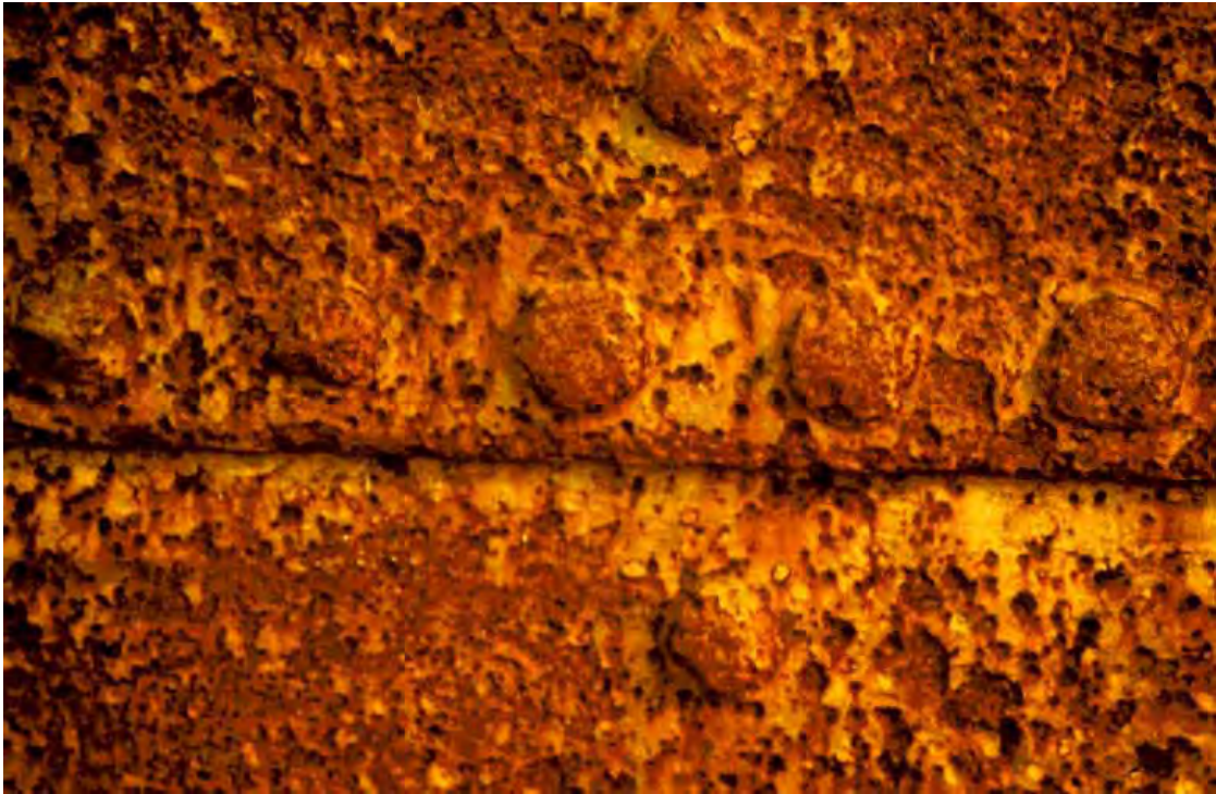
Fig.9: Riveted construction of the English dredge in the Berleg Goldfield. Note severe corrosion pitting.
