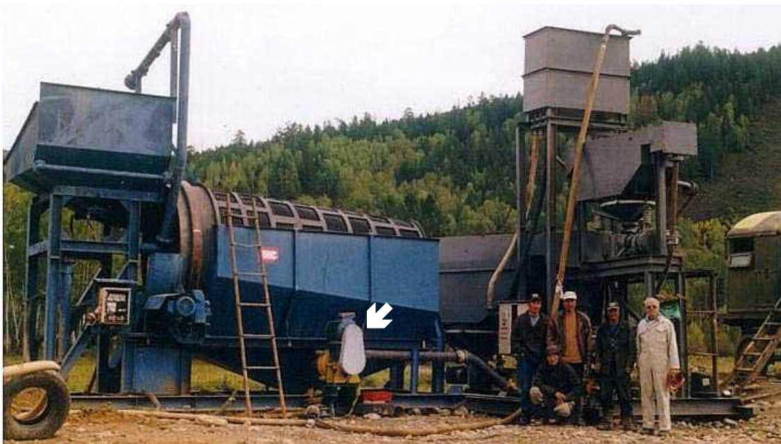
Fig.11: Frank M c Bride (right) with team at the Bugant Mine, having completed the electrical wiring of the IHC 2-Cell Jig (right) and the IHC Conical Screen (left). Note the Warman Pump (arrow) for pumping slurry by pipeline from the screen to the jig.
