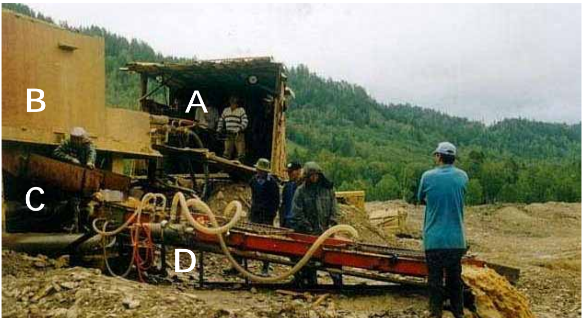
Fig.10: A Russian water cannon 'monitor' (A) blasting pay-gravels above a static screen (B), feeding slurry via a link chute (C) to the 25m 3 /hour PAuSE NZ Hydraulic Riffled Sluice (D).
